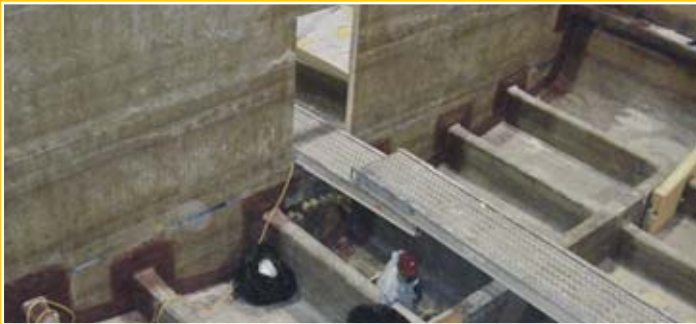
A web frame and a freshly landed bulkhead support the bottom girders
