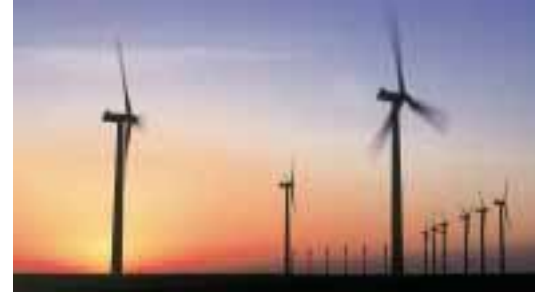
Wind energy establishes itself as a reliable and clean form of energy in wide areas of the world.
